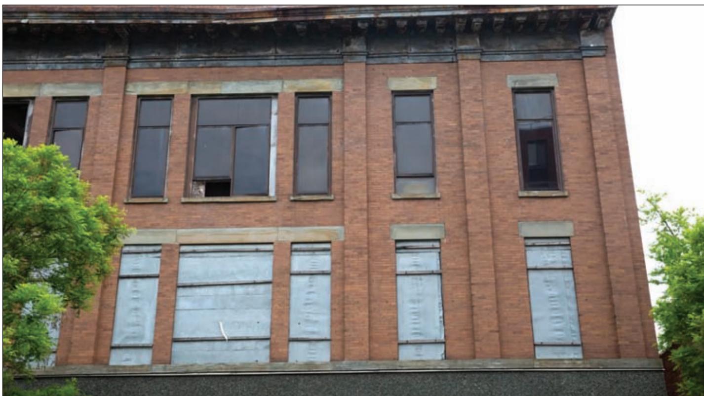
Boarded-up windows at 1024 Fulton Street.
