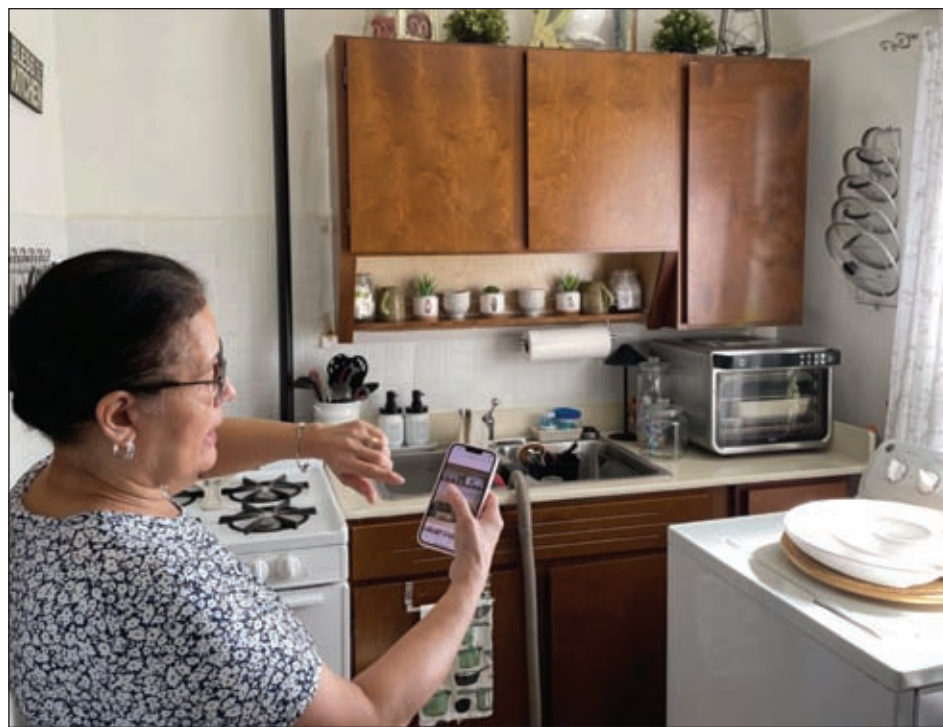
Jacob Riis Houses tenant Blanca Ramos shows where a kitchen cabinet fell from her wall after a water leak. April 15, 2024. Credit: Greg Smith/THE CITY
